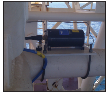
Helideck Motion Monitoring
